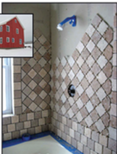
Tile work on Creamery Road in Egremont. Shower features 2 shower heads and custom tile work by CBS - Bob Smith
